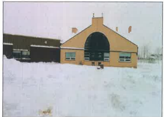
Pooling occurs on the site at the South moduls during spring thaw. Lighting levels should also be improved in this area.
