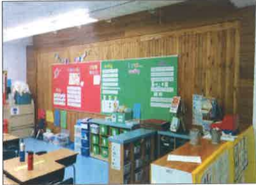
Noise transfer is an issue between classrooms 105 and 102 due to the stage opening being infilled.
