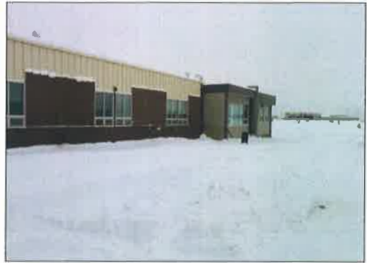
Supervision and lighting level is an issue on the North side of the modular classrooms.
