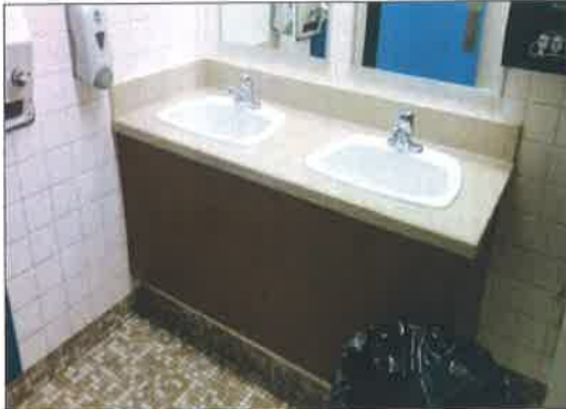
Upgrades are required in the washrooms to meet current barrier-free guidelines.
